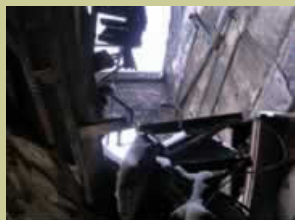
Hurt room: looking up in the room where the ceiling collapsed; the sky looks grey here
