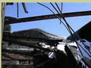
Kerr Roof: where the fire started, looking up through the non-existent roof
